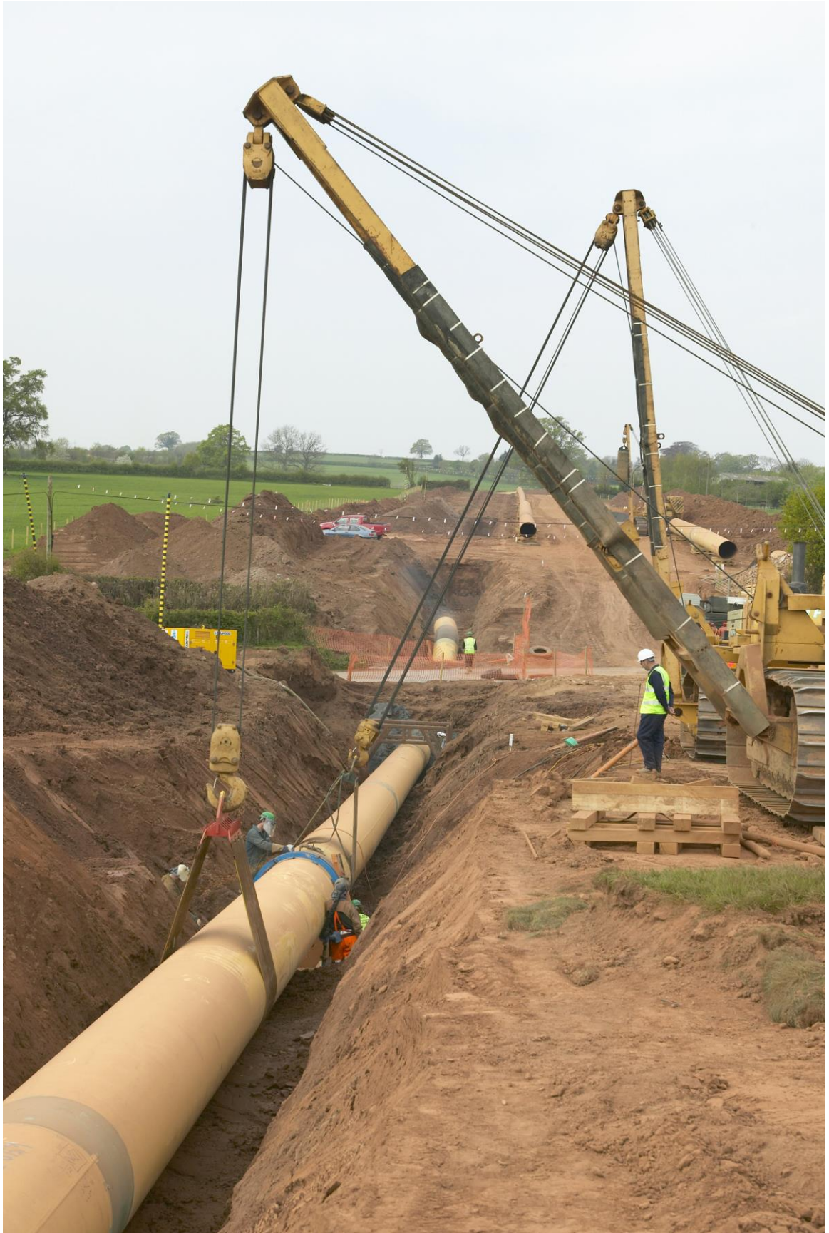
3.11 Image showing a pipeline spread with obstacle crossing. The additional land here has been consumed predominantly by excavations and soil.
